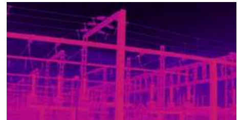
Automatic temperature control system based on high accuracy thermography
